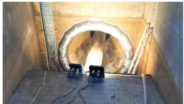
Figure 3: A VETT turbine during installation at Eaton Socon, Cambridgeshire in the UK.
