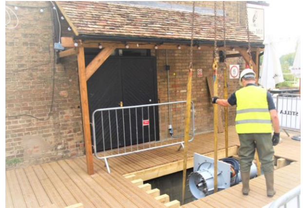
Figure 2: A VETT turbine during installation at Eaton Socon, Cambridgeshire in the UK.
