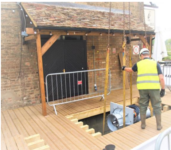
A VETT turbine during installation at Eaton Socon, Cambridgeshire in the UK.
