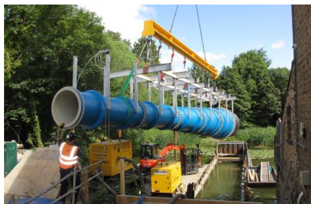
Visual 1: GRP Venturi pipe, hung into water from frame
